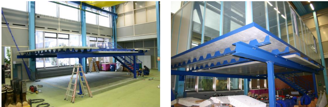
Figure 10 – New platform built using the novel type of composite slab system for a work space located in the ETH testing laboratory
