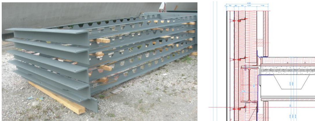
Figure 9 – Steel beams with angles as supports before concreting (left) and detail of the facade at the residential building “Residenza Villa Lugano” under construction (right)
